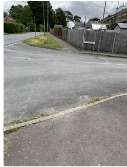
Photograph 14: Crossing infrastructure along Hillbury Road
