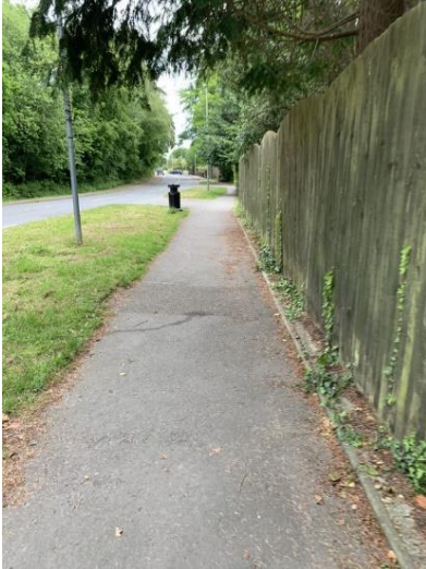
Photograph 1: Footway along Station Road
